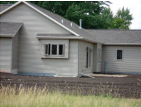
Figure 1: Radon Mitigation System view from the outside.
